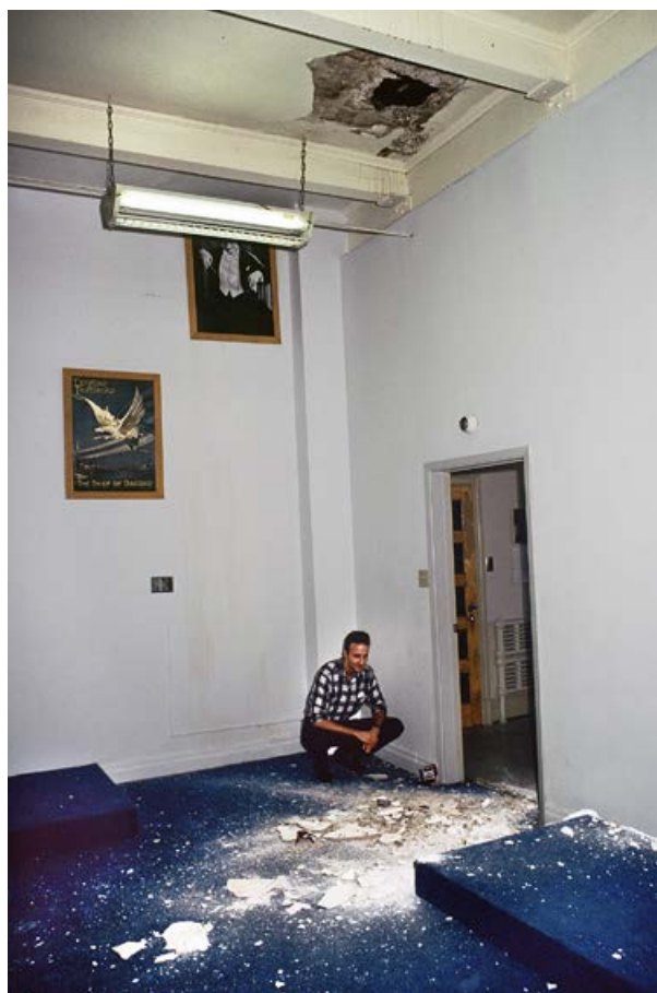
My friend Phil Spurrell in the Montreal studio, 1994, after a chunk of the ceiling collapsed from water damage. We'd laugh, clean up the rubble, and set up more of the tarp drainage system. The art on the walls was hung to cover other damage
